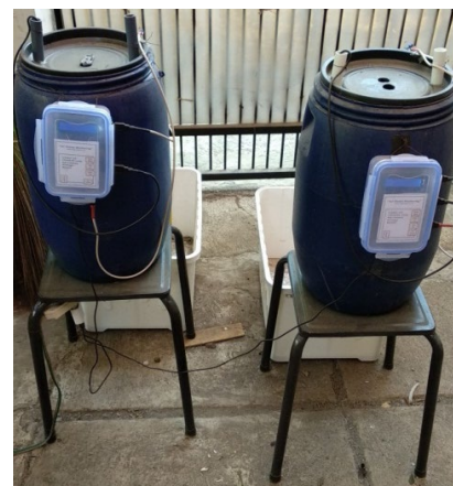
2: Installation of an irrigation tank monitoring system
